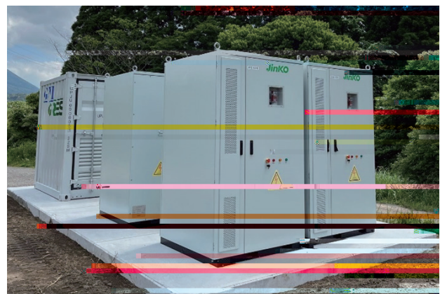
Fig. 2 Jinko ESS 215kWh DC Blocks
